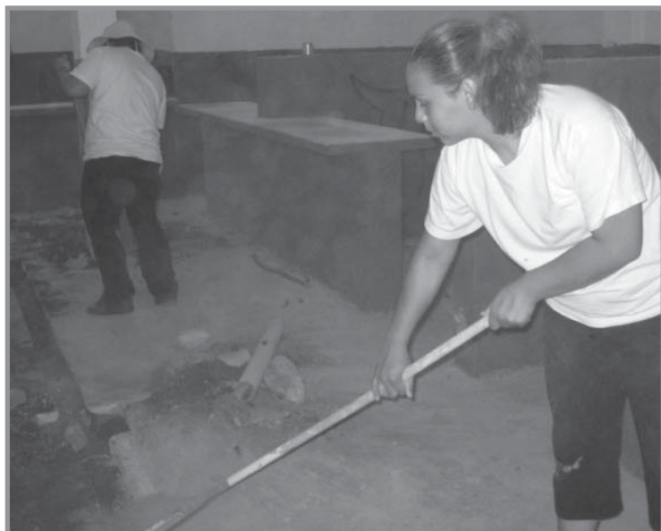
Katrina Carranco, pictured in front, and sister, Araina Carranco, helped clean-up after they layed plumbing for the San Andres marketplace.
