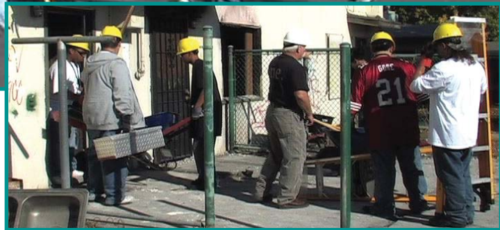
Pictured above are YouthBuild San Joaquin students as they reconstruct a fire-damaged building as part of their community improvement project.
